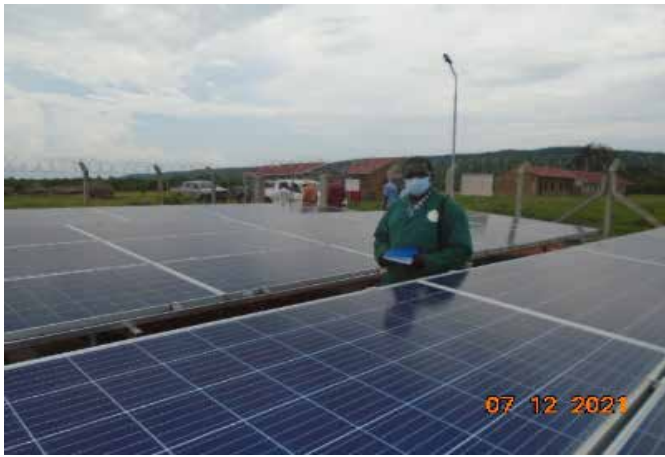
Figure 8: Solar off-grid in Kasese
