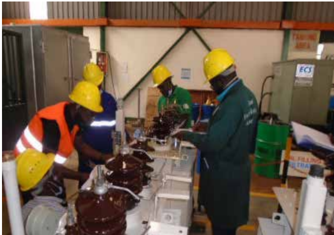
Figure 5: FAT for transformers at ECS, Kawempe
