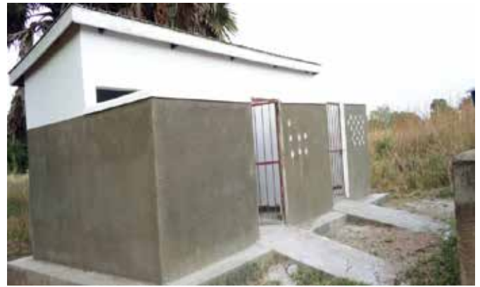
Figure 3: A 4-stance drainable pit-latrine at Pajimo Primary School
